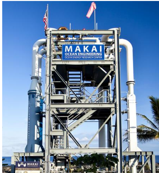
Figure 1-4: Makai OTEC power plant in Hawaii. Source: https://www.makai.com/ocean-thermal-energy-conversion/
