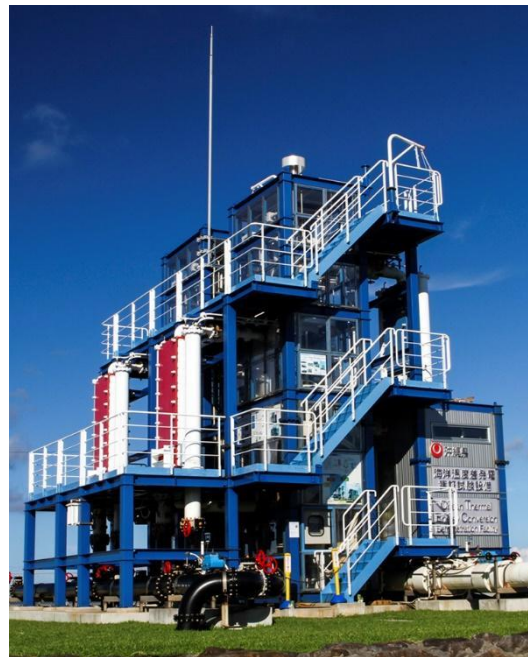
Figure 1-2: 100 kW power plant in Kumejima: source: http://otecokinawa.com/jp/index.html .
