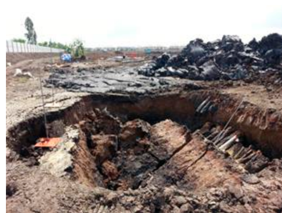
Fig. 13. Failure of type E soil cement wall at excavation depth of 5 m.
