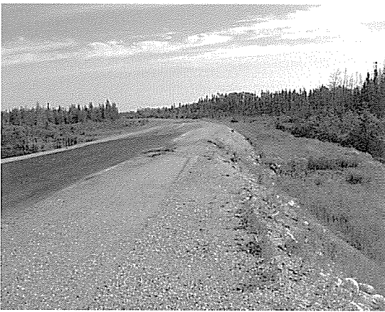
Fig. 2 Road embankment in Northern Manitoba showing signs of lateral movements and differential settlements (courtesy of Manitoba Transportation and Government Services)
